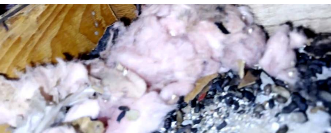
ENTIRE KITCHEN CRAWLSPACE FILLED WITH RODENT FECES
