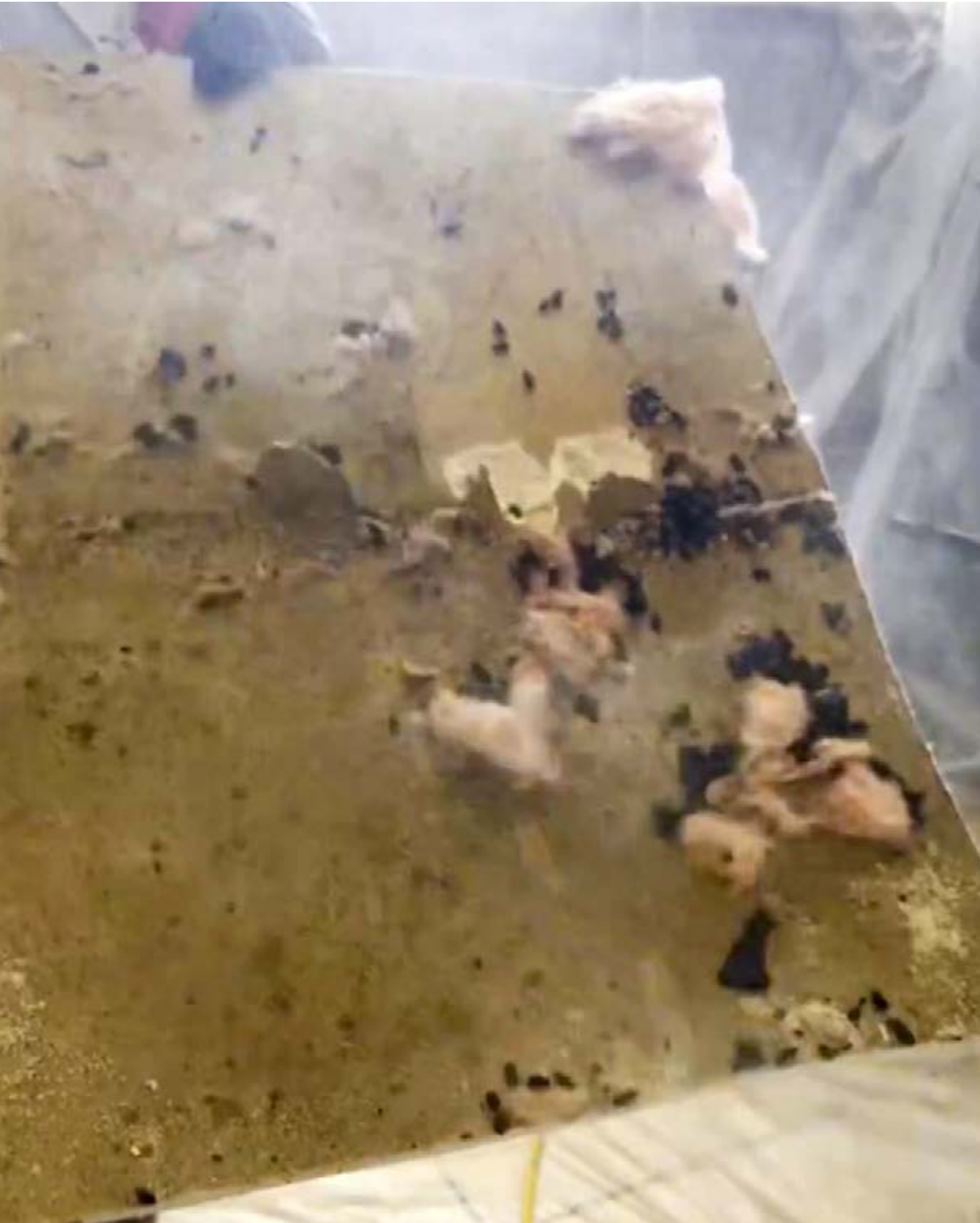
DRYWALL AND INSULATION SOAKED WITH URINE AND FECES
